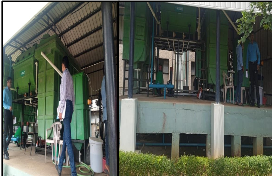
STP unit in SKASC, Coimbatore, Tamil Nadu
